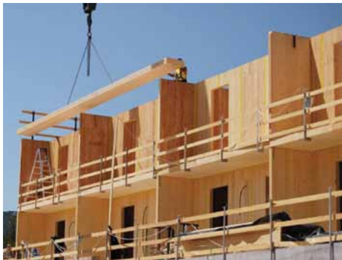
Prefabrication of timber buildings dramatically reduces construction time and cost by enabling much of the preparation to be undertaken in weather-tight conditions offsite.
