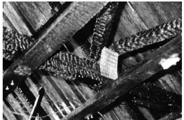
Poor fire performance of an unprotected tooth-plate connection
